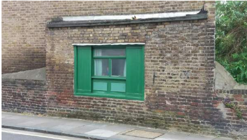
Serving hatch. Flank elevation of no. 1 Faroe Road on to Milson Road.
