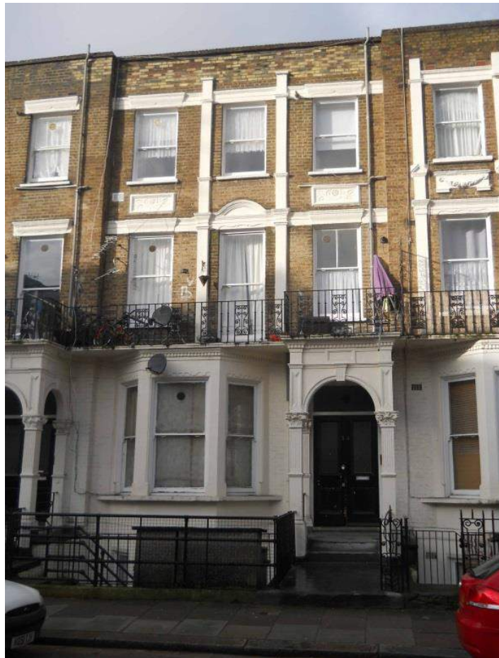
20-36 Hazlitt Road. Missing cornices diminish the decorative composition.
